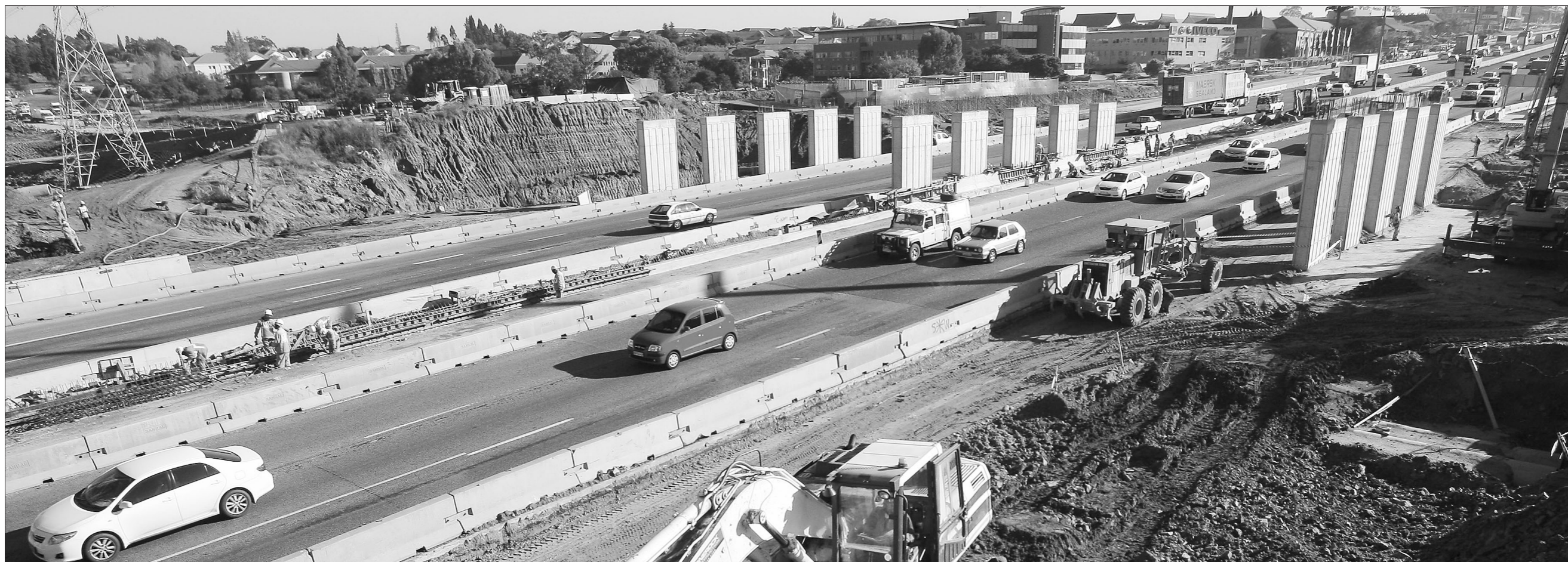
Road race: the Allandale slip road in Johannesburg just six weeks before the World Cup was due to start. Crews worked through the night to finish before the event
