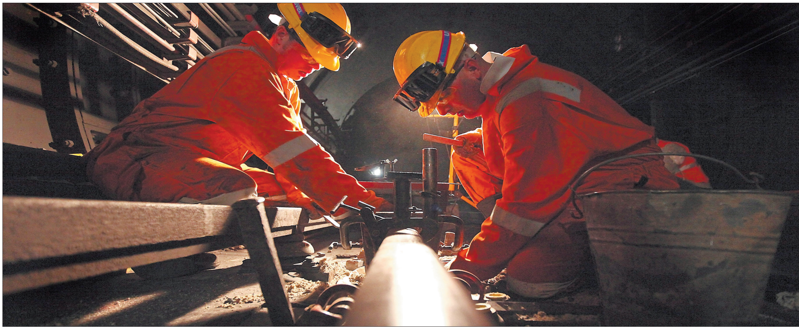
Going underground: workers prepare to improve London Underground infrastructure while minimising disruption to services
