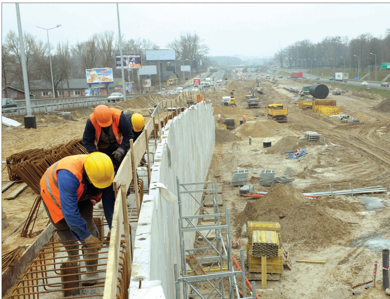
Road to ruin or salvation? A consortium including Chinese interests is working on Poland's east-west highway
