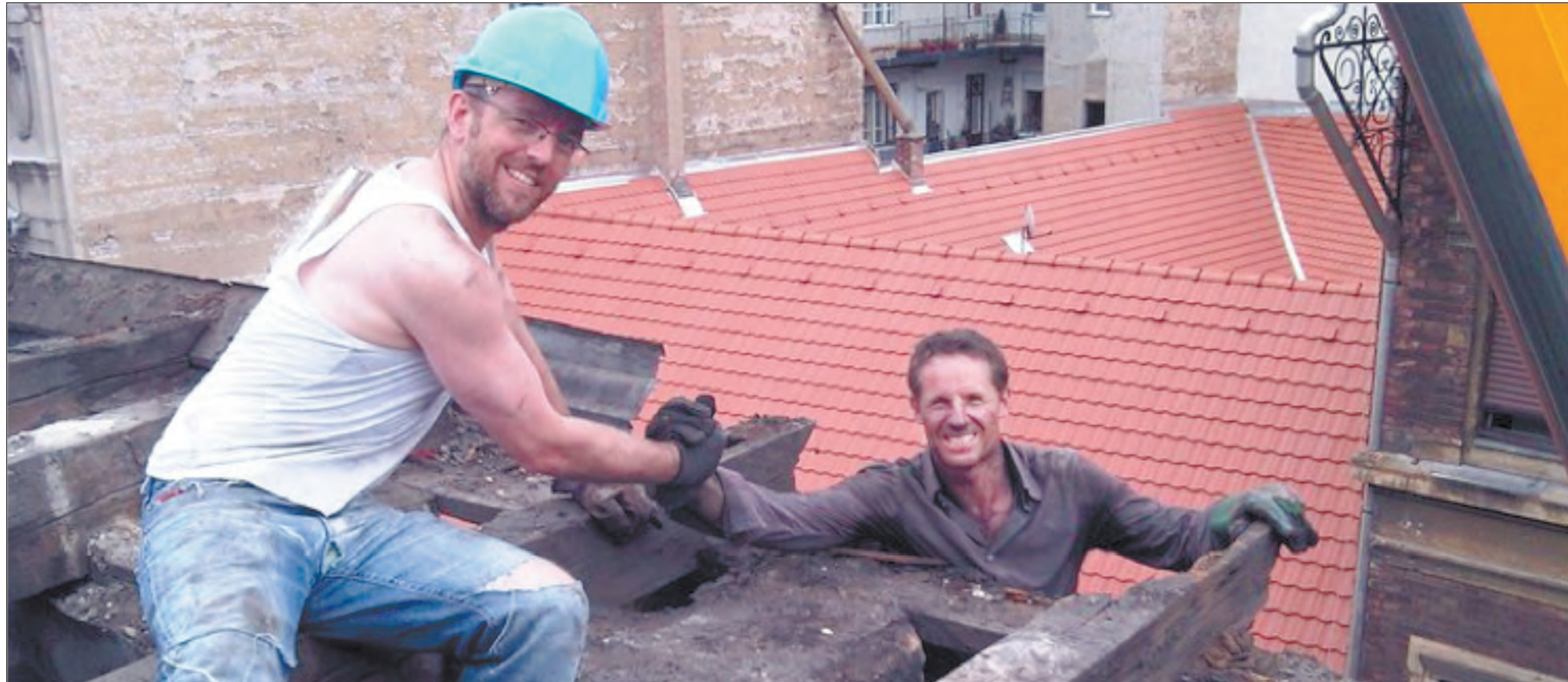
Up on the roof: business partners Peter Grundberg, left, and William Clothier take a hands-on approach to restoring and renovating one of their properties
