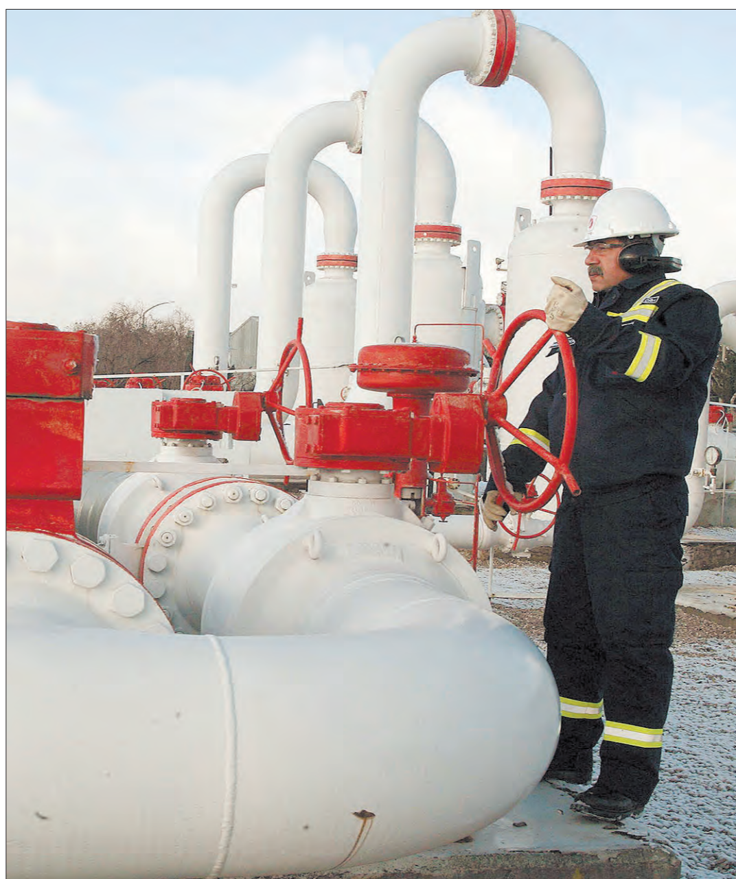
Supply lines: routine checks are carried out at a natural gas control centre west of Ankara. A new gas pipeline is planned for 2018
