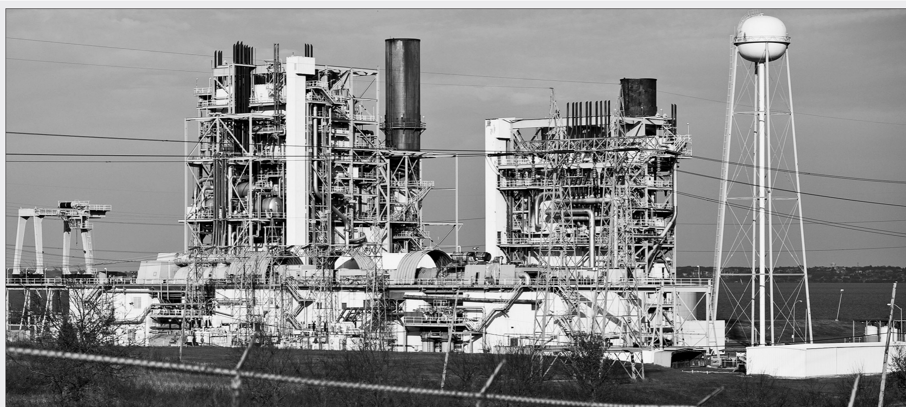
Price-sensitive: EFH subsidiary Luminant's natural gas power plant at Lake Hubbard, east of Dallas, Texas
